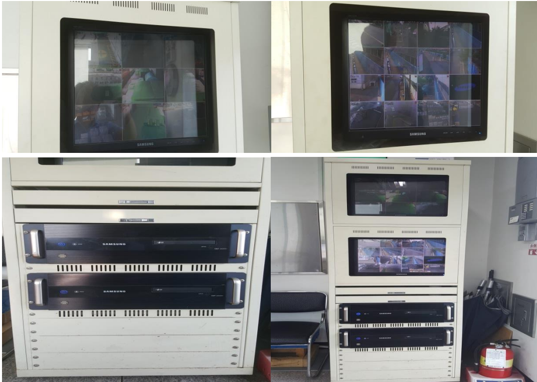
<CCTV monitoring in Security office>
